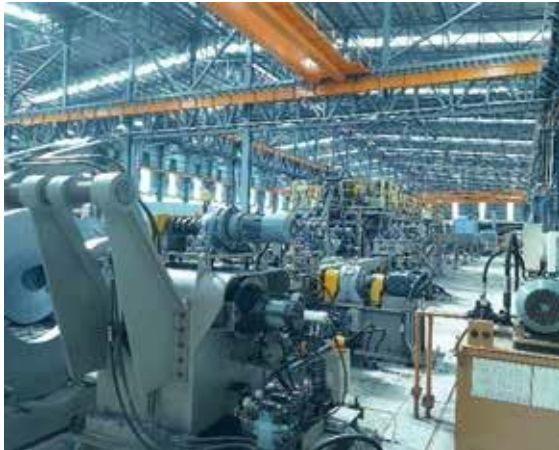
H-Beam Line view From Uncoiler
